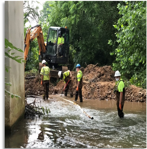
Crews make an emergency sewer repair along Milligan Hwy at the intersection of Powder Branch Rd.
