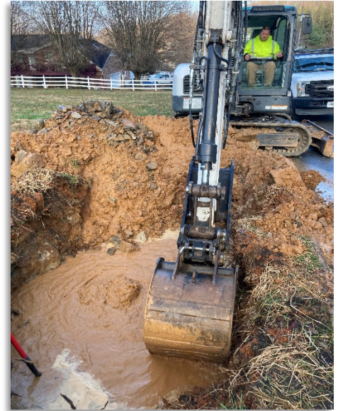
Main line leak repair on Westwood Street that was identified by the leak correlator.
