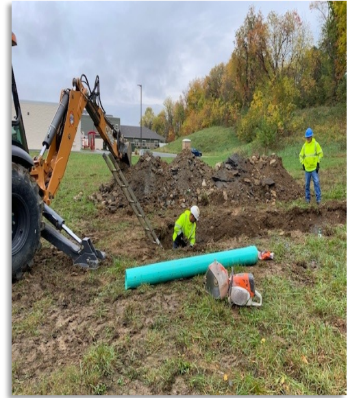
Sewer personnel complete a line repair to allow access for investigation near Williams Avenue.
