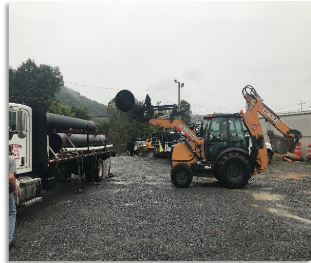
Receiving and unloading the 24" ductile iron pipe for the State Park sewer repair.
