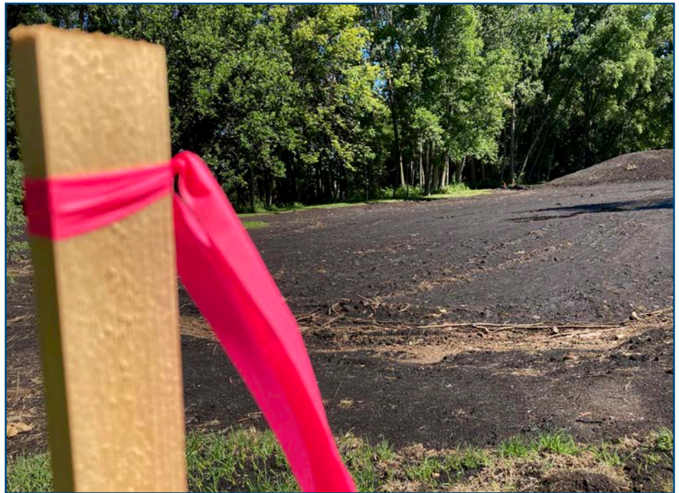
A line of vegetative debris marks how high the water reached in a newly constructed wetland after a rain the day before. The wetland, built on city-owned property bordering a ditch in Winsted, will filter about 15 acres of residential stormwater runoff bound for Winsted Lake. The project, a collaboration that included the McLeod SWCD and the city of Winsted, was nearing completion on Aug. 15, 2023. Photo Credit: Ann Wessel, BWSR
