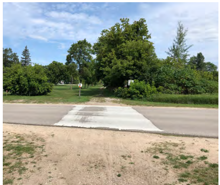
Existing striping/coating at road crossing
