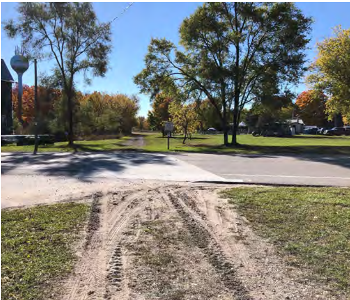
Example of loose/sandy trail surface material
