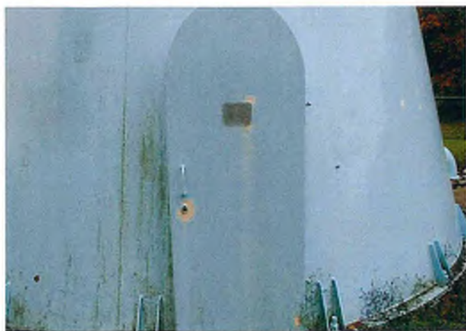
Tank Access Door Locked
