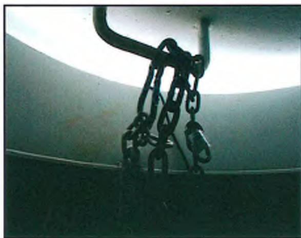
Secured Roof Access Hatch
