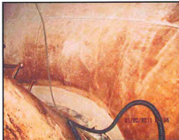
Interior area after washout.
