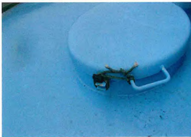
Wet Interior Access Hatch Locked
