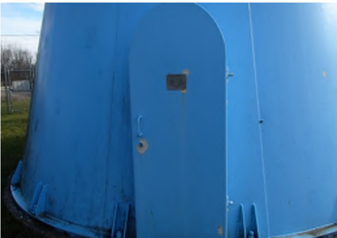
Tank Access Door Locked
