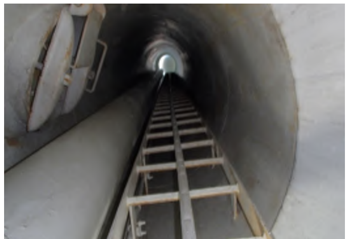
Dry Interior Coating Dry Riser
