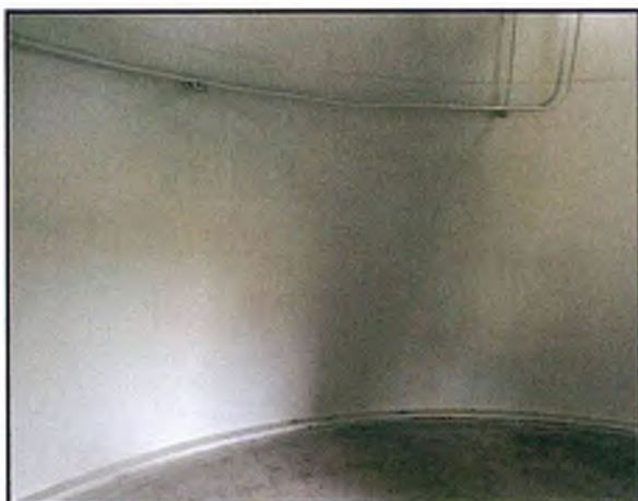
Dry Interior Foundation
