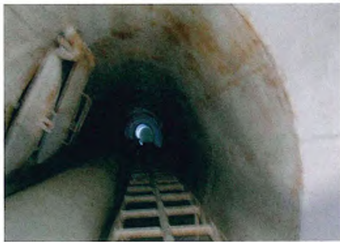
Dry Interior Coating Dry Riser
