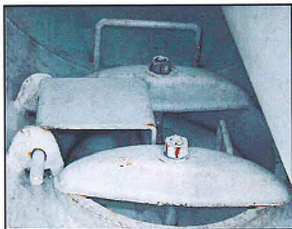
Shell manway is secure.
