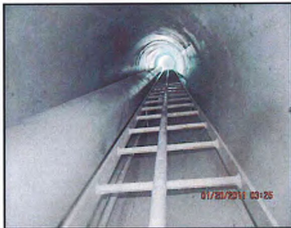
Access ladder equipped with safety climb.
