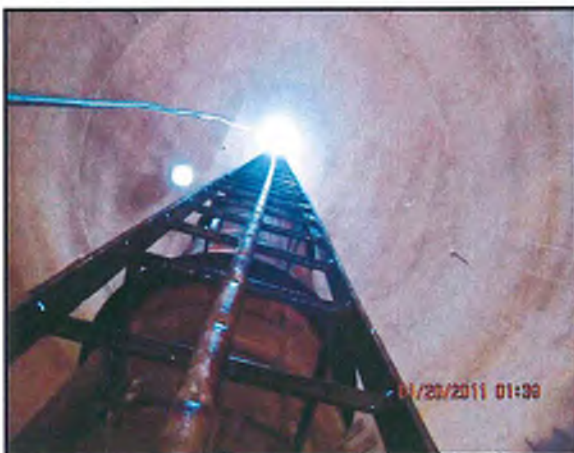
Interior area after washout.
