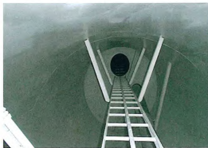
Safety Climb on Access Ladder
