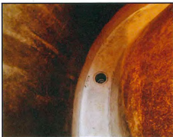
Interior Floor (Post-Washout)
