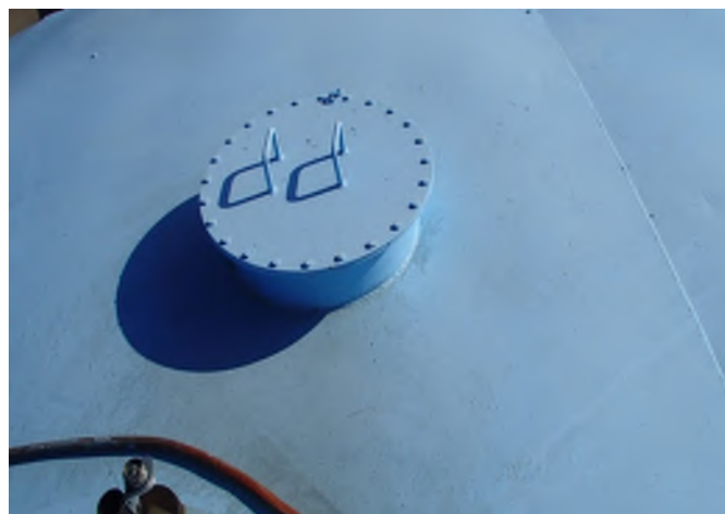
Bolted Wet Interior Bolted Hatch
