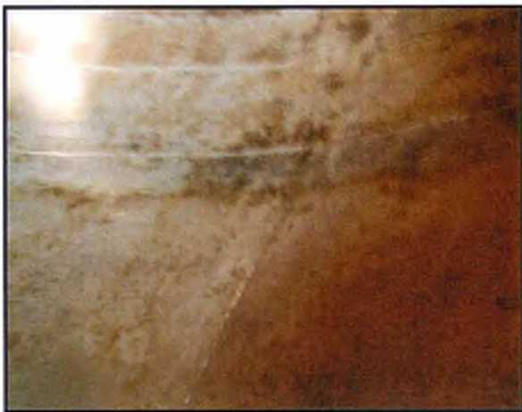
Interior Sidewall (Post-Washout)
