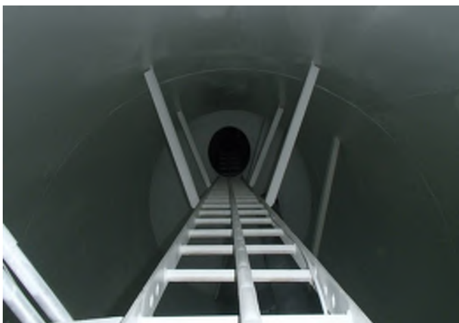
Rigid Rail on Access Ladder
