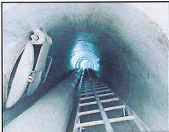
Access ladder equipped with safety climb.
