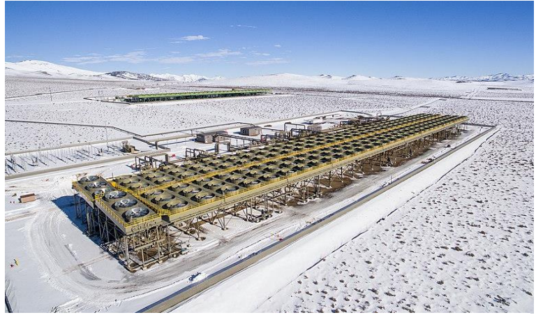
McGinness Hills Geothermal Plant | Source: Nevada BLM
