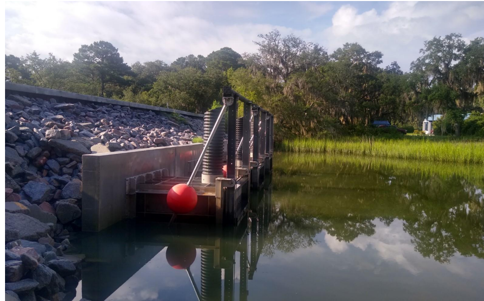
Figure 5.15. Example of Muted Tide Gate installed in Beaufort, SC
