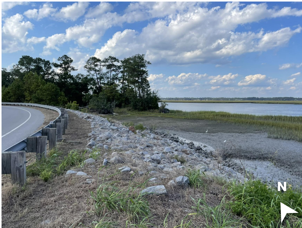
Figure 4.7. Site photo of guardrail and road-adjacent revetment along the Hwy US-21 westbound lane of the underpass
