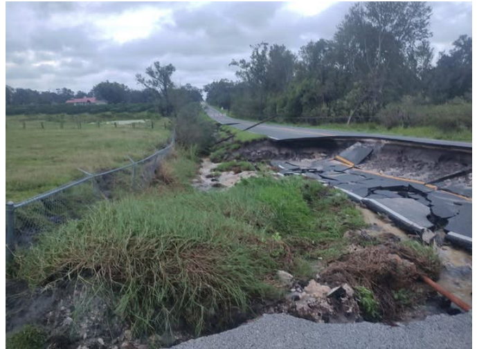
Figure 23: Curley Road damage after Hurricane Milton
