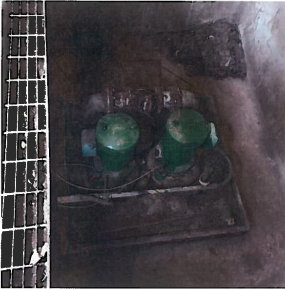
Image 5. Recessed floor and pump skid.
