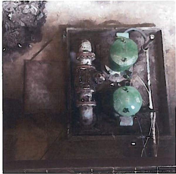
Image 6. Pump skid and access hatch.
