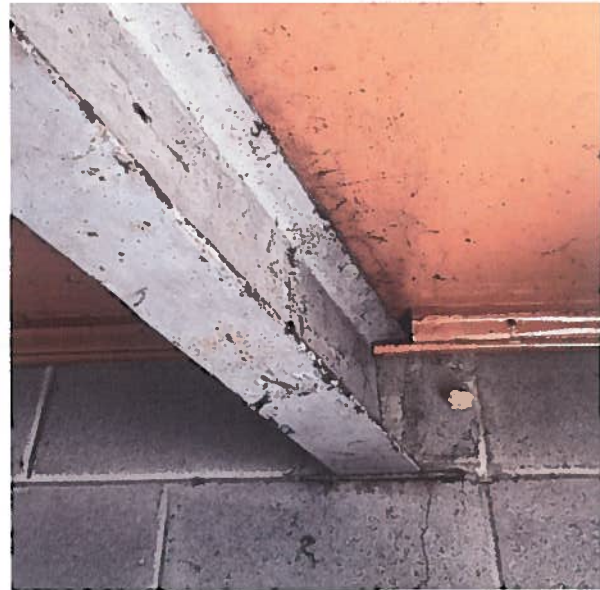
Image 8. Trolley hoist beam.
