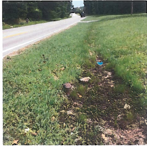
Image 10. Emergency pump connection.
