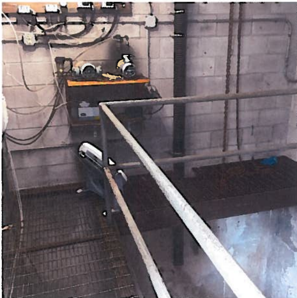
Image 3. Pump station interior.
