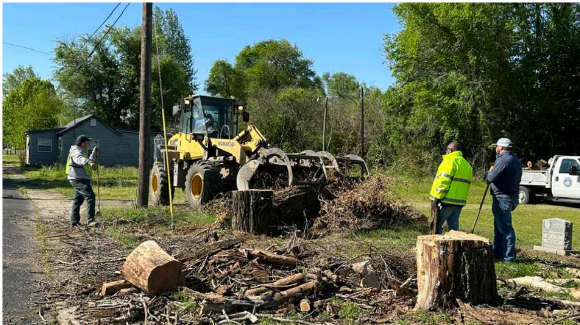
Community Development helped remove remaining tree debris from the Sunset Cemetery in May.
