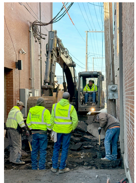
Milling and resurfacing was done to the downtown alley between Front and Center Street as part of the 2023 Street and Drainage Improvements Program.
