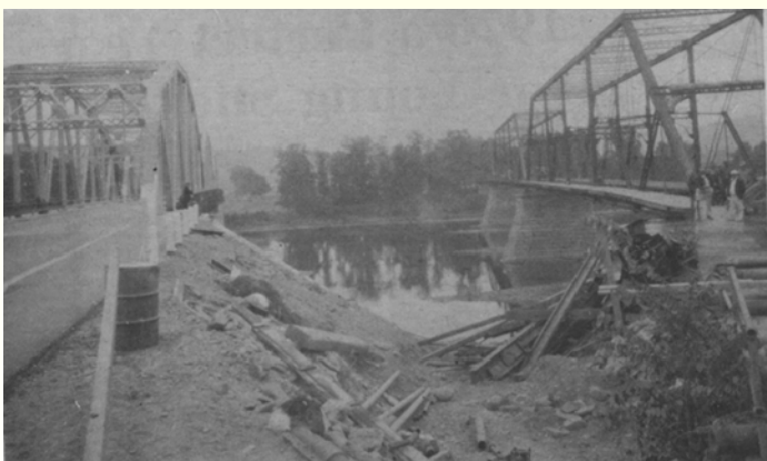
Looking south; the 1936 Bridge on the left, the 1895 Bridge on the right just before demolition.
