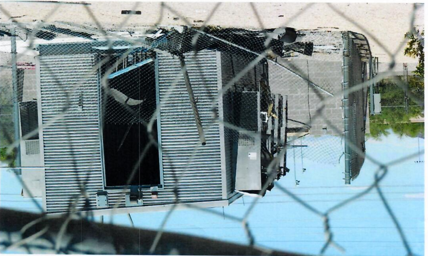
View of debris and damage to the rear door, HVAC systems, and the container. PHOTO: ARIZONA PUBLIC SERVICE
