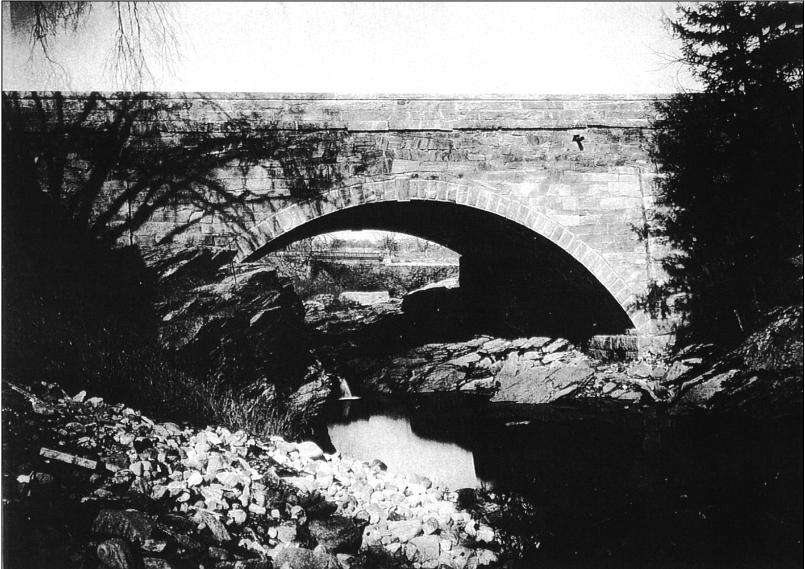
Figure 1: A beautiful cut stone bridge over the Ware River near Downtown Ware
